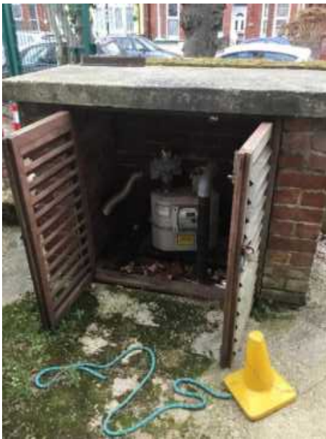
Gas isolation and meter, main school and boilers, Ludlow Road side, near to playground corner and Year 3 doors and fenced gate
