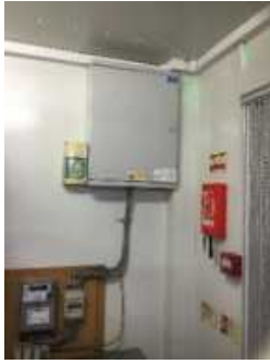
Electric isolation and meter, kitchen pod, dedicated supply, not on older plans
