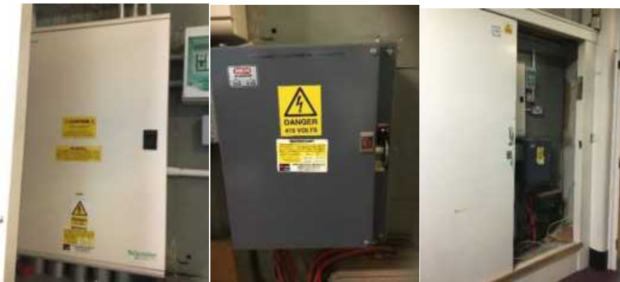
Electric isolation and meter, main school, link corridor, between reception and Year 3
